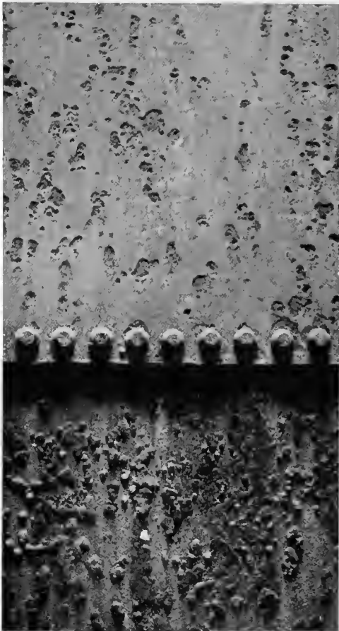
Lower part, rust lumps, or "tubercles"; \times \frac{1}{8} . Above, part of the same surface, sand-blasted, showing pitting
